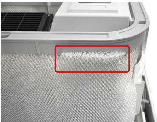
Fig. 6.3.2.5: Incorrect fit of the filter
